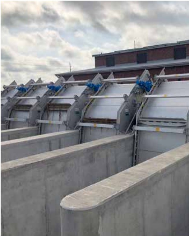
Several HUBER Coarse Screen TrashMax® loaded in parallel.
