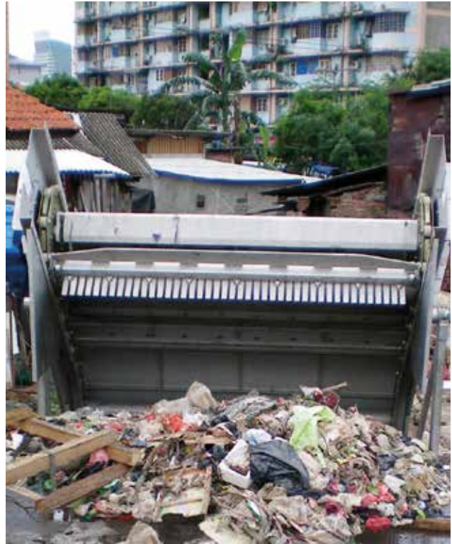
Free discharge of the screenings prevents blockages.
